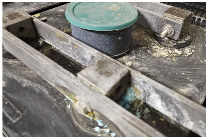
Corrosion was discovered on #55.
