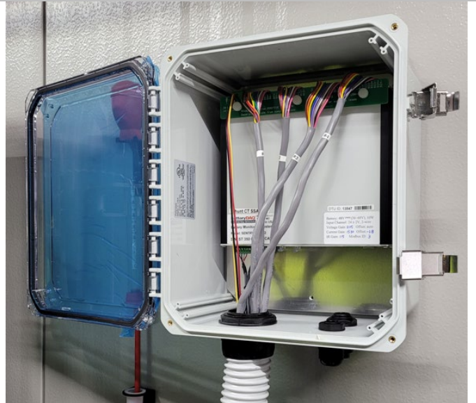
Mounted on wall directly without Unistrut
