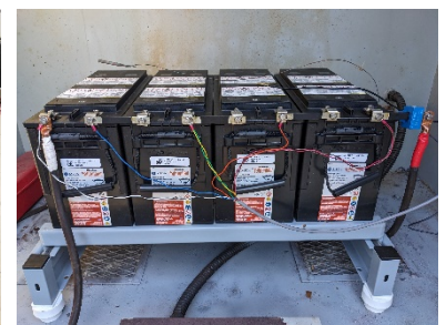
Substation Support System
