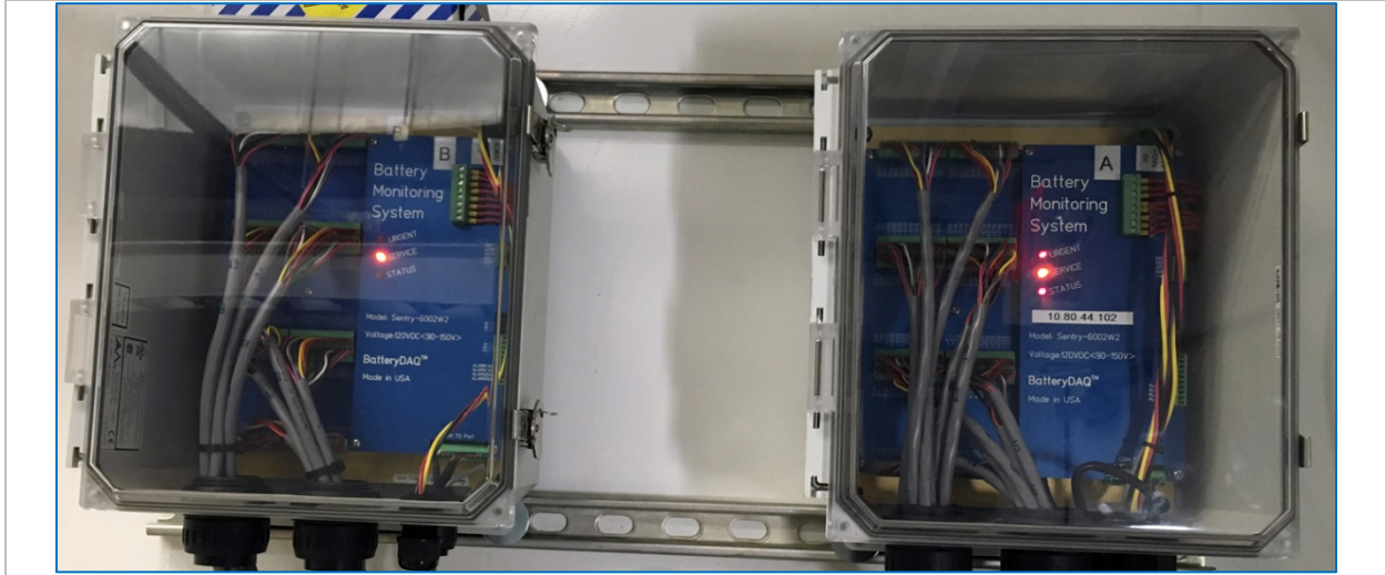
Mounted on wall with Unistrut
